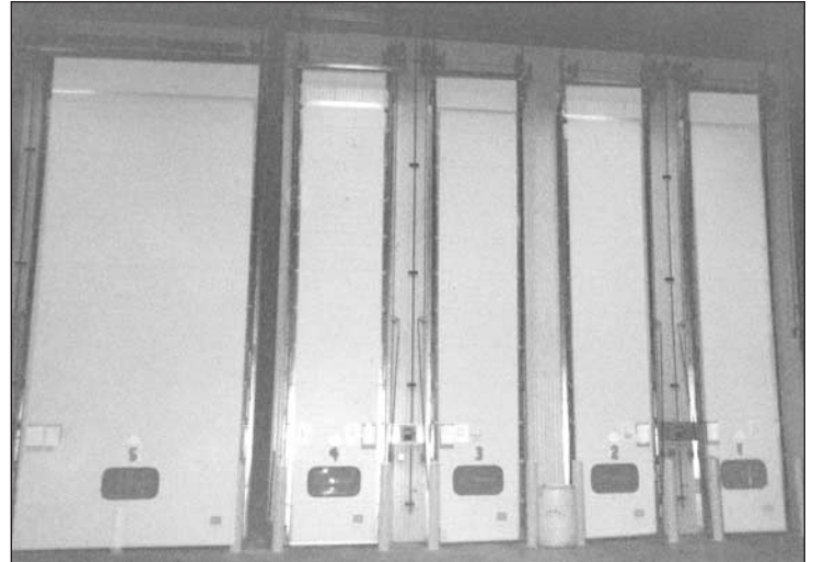
Five new TARPLESS® single- and double-wide ripening rooms inside the new low-temp addition at the Roundys D.C. in Westville, IN.
